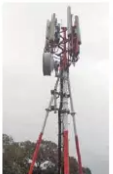
Newly established highly quality voice and 4G base station.
