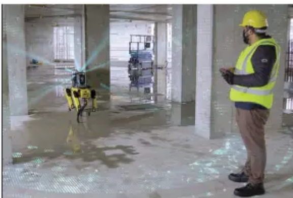
Spot can effectively scan and monitor progress of construction, saving up on time and money.
