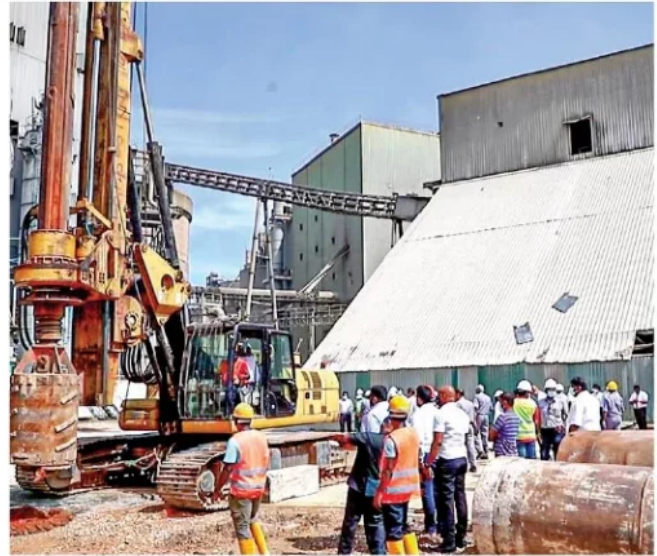
Tokyo Cement Group's factory expansion project in Trincomalee will add another 1 million metric tons to its production capacity.
