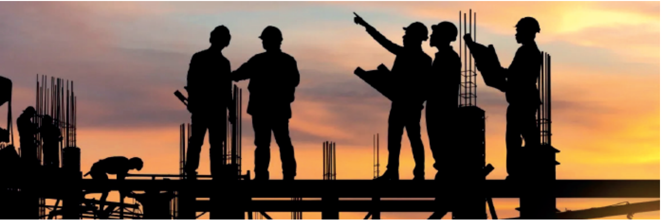
Construction in progress taking place across many places for AI Data Centers,
