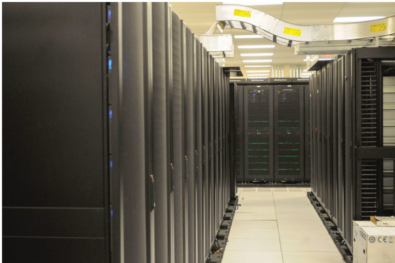
NERSC data-center racks.
